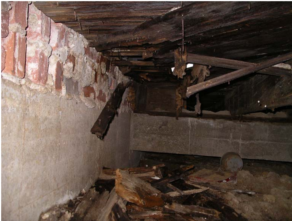
#5760 – Fire damage is quite localized.
