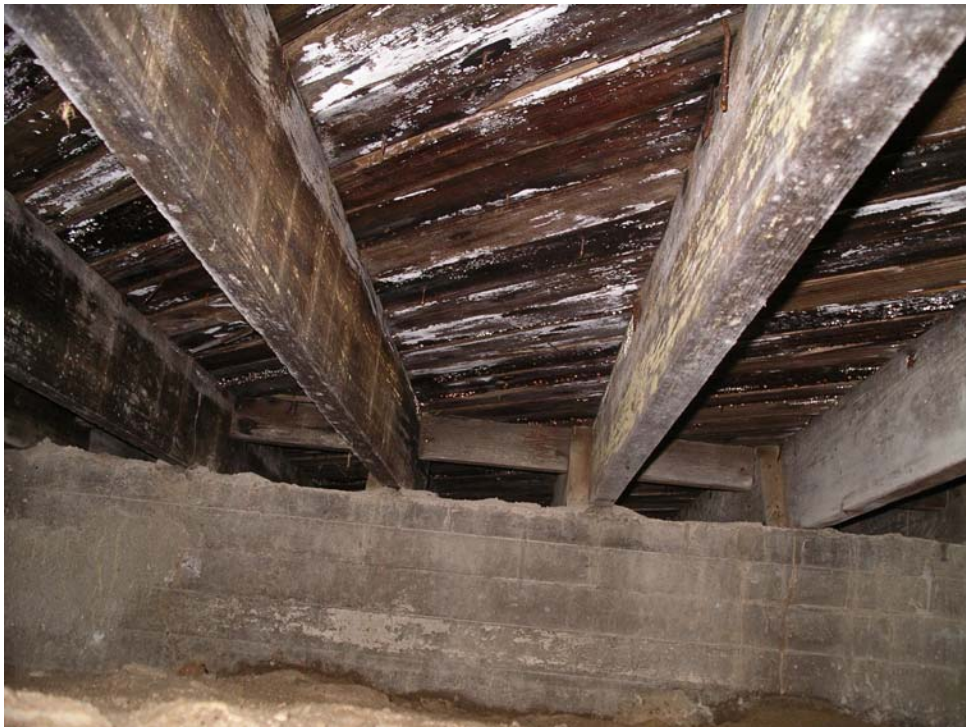
#5751 – Extreme humidity has caused moderate damage to the floor structure.
