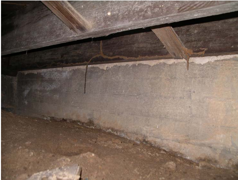
#5743 – Evidence of past termite presence may indicate damage.
