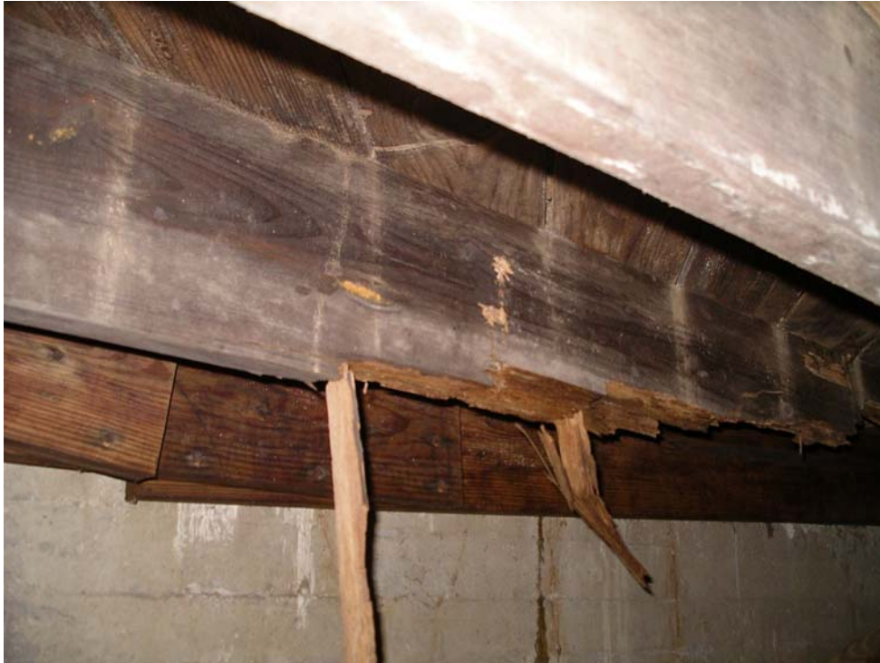
#5636 – There is isolated damage to floor members.
